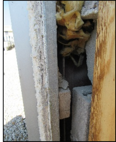
↑ Single pane layered stucco walls poorly insulated
