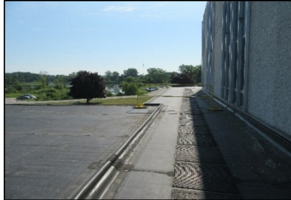
↑ No fall protection in areas of the roof
