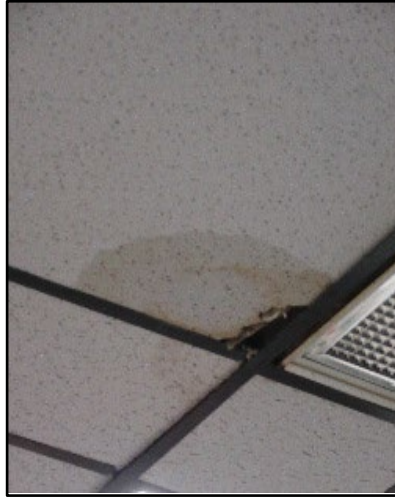
↑ exterior brick leaks causing water intrusion
