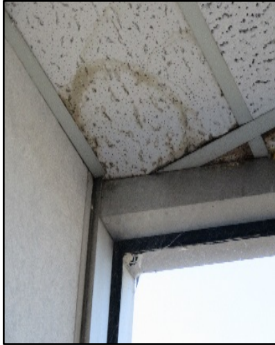
↑ Single pane windows leaking water and air
