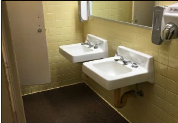
↑ Outdated bathrooms that are not ADA compliant
